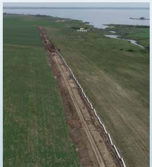
Raw Water Parallel Pipe from Intake to OMND
