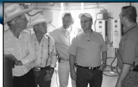
From left: Morton County Commissioner, Jim Boehm; SWA Director, John Klein; Morton County Commissioner, Bob Christianson, SWA Director Larry Ziegler and Bartlett & West Construction Administrator, Bob Keller tour SWPP construction in Morton County.
