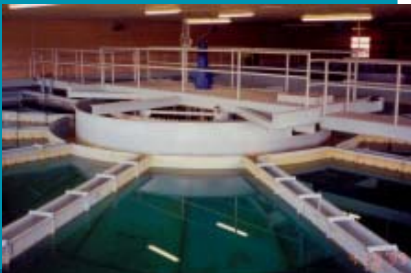
System Water Treatment Plant located in Dickinson, North Dakota.
